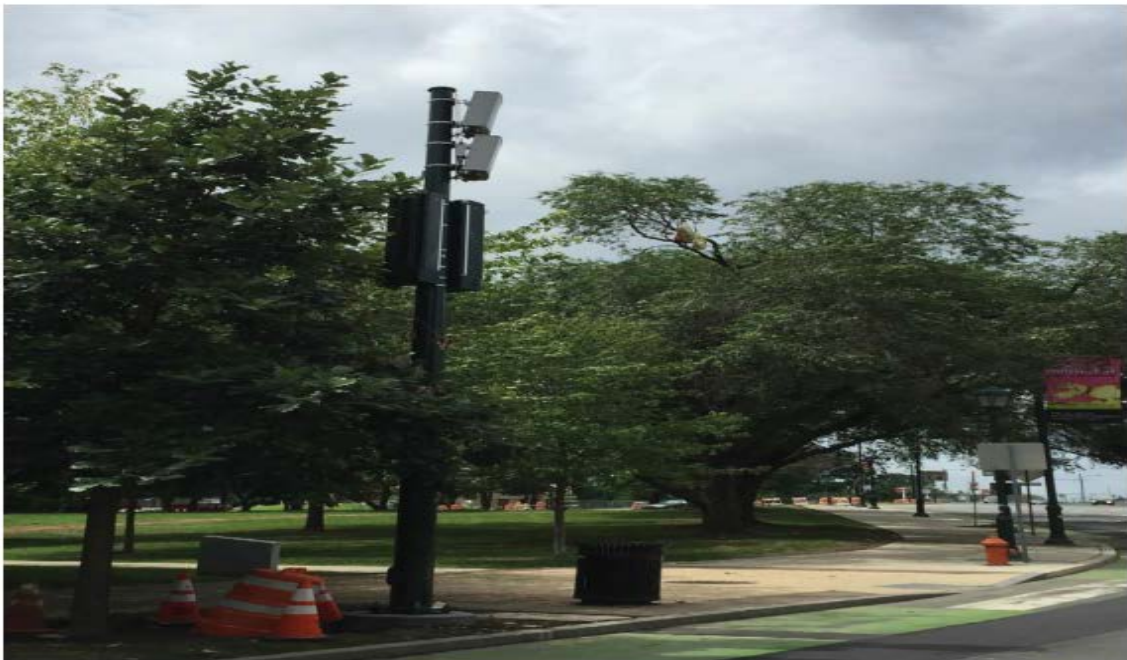
Figure 16. Crown Castle small facility deployed in historic district on Benjamin Parkway, Philadelphia, PA 16
